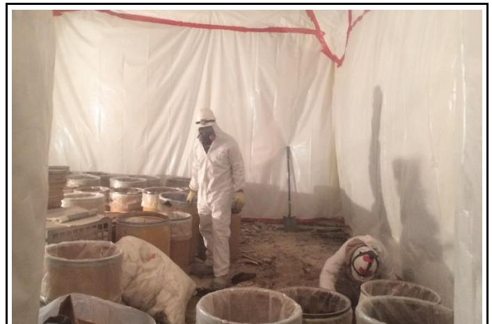
Asbestos abatement work to support the I-95, Section BSR project in Philadelphia, Pennsylvania
