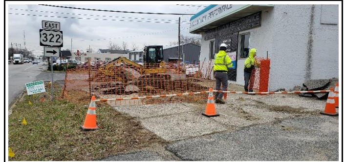
Photograph showing the placement of orange safety fencing (i.e., barricade) around an open excavation for the removal of two USTs for the PennDOT S.R. 0322 Improvements Project in Delaware County, Pennsylvania
