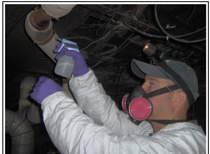
Collection of asbestos samples, City of Lebanon Bridge Street Project in Lebanon County; PennDOT Engineering District 8-0
