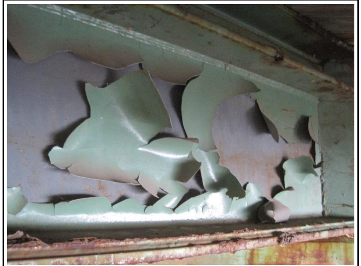
Photograph taken during a LBP inspection of a bridge along S.R. 3016 in Canton, Bradford County, Pennsylvania
