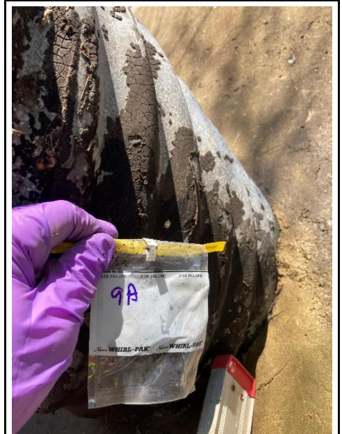
Sampling of suspect asbestos-containing tar from outside of a corrugated drainpipe associated with a concrete bridge abutment, S.R. 00011 Bridge over Conodoguinet Creek in Cumberland County, Pennsylvania
