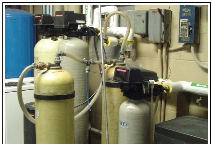
Water treatment system at the PennDOT Bear Creek Maintenance Facility, Engineering District 4-0
